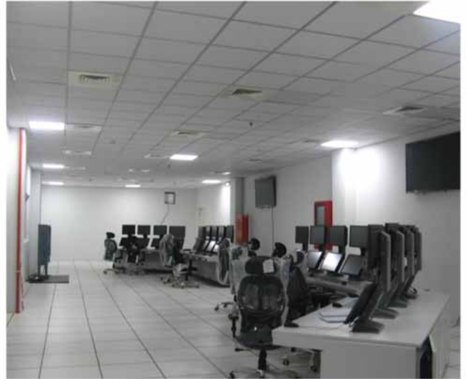
CONTROL ROOM DCS
