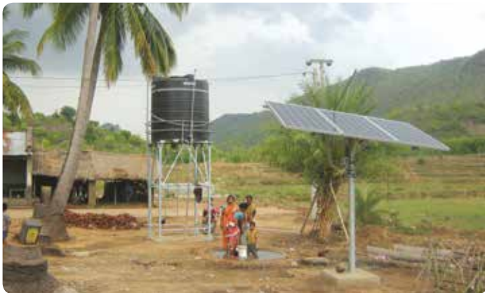
Solar hand pumps installed in rural and backward areas in Orissa for drinking water purposes. Water is lifted into overhead storage tanks during daytime using solar power.
