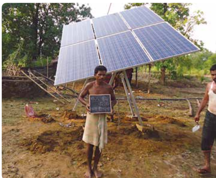
2HP Solar submersible pumps for irrigation purposes installed in remote, tribal inhabited area in Gadchiroli District, Maharashtra.
