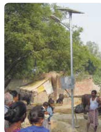
About 18,000 Solar street lighting systems were installed in remote and poverty stricken villages in Uttar Pradesh.
