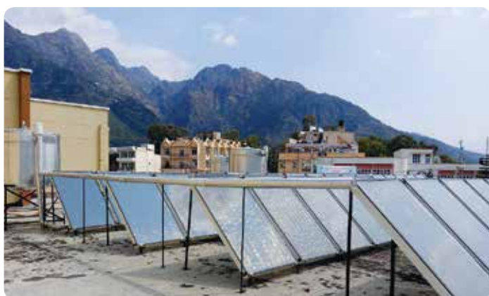
Installation of 1,34,000 lpd (litre per day) capacity Solar Water Heating Systems at various Bhakta Nivas and Dhams of Shree Mata Vaishno Devi Shrine Board, Katra, Jammu.
