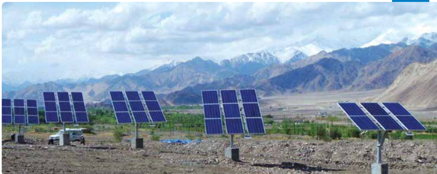
Solar powered pumps for sprinkler irrigation, installed at Leh, J&K. These pumps in the Himalayan Ranges are the highest such installations in the world.
