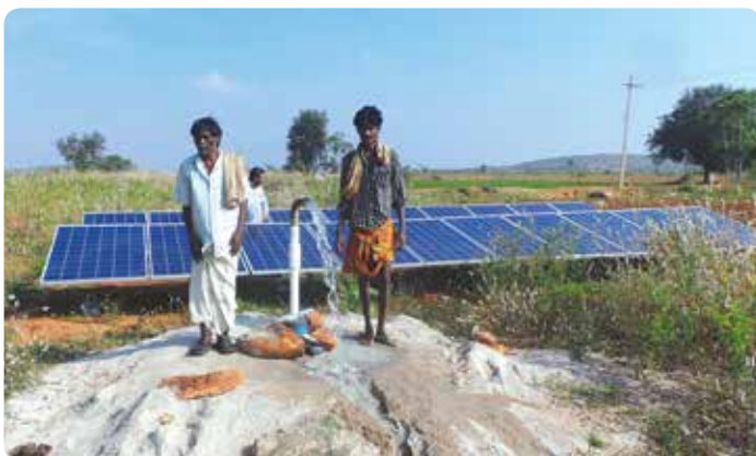
5HP AC Solar submersible pumps for irrigation purposes installed in Karnataka.
