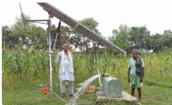
2HP Solar surface pumps for irrigation purposes installed in Bihar.
