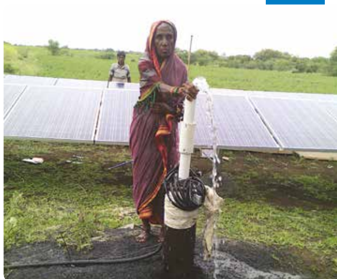
5HP AC Solar submersible pumps for irrigation purposes installed in Karnataka.
