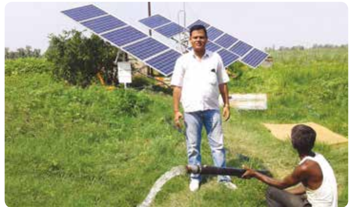
3HP DC submersible Solar water pump for irrigation purpose installed for marginal farmers in Uttar Pradesh. This gives the farmers much needed relief from dependence on diesel engines.
