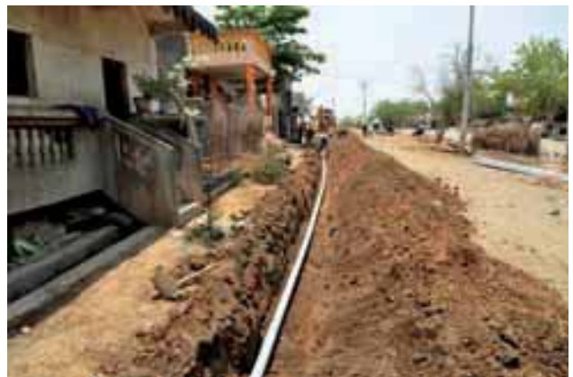
Conveying water; laying a pipeline in the Shirsoi Panchayat for drinking water
